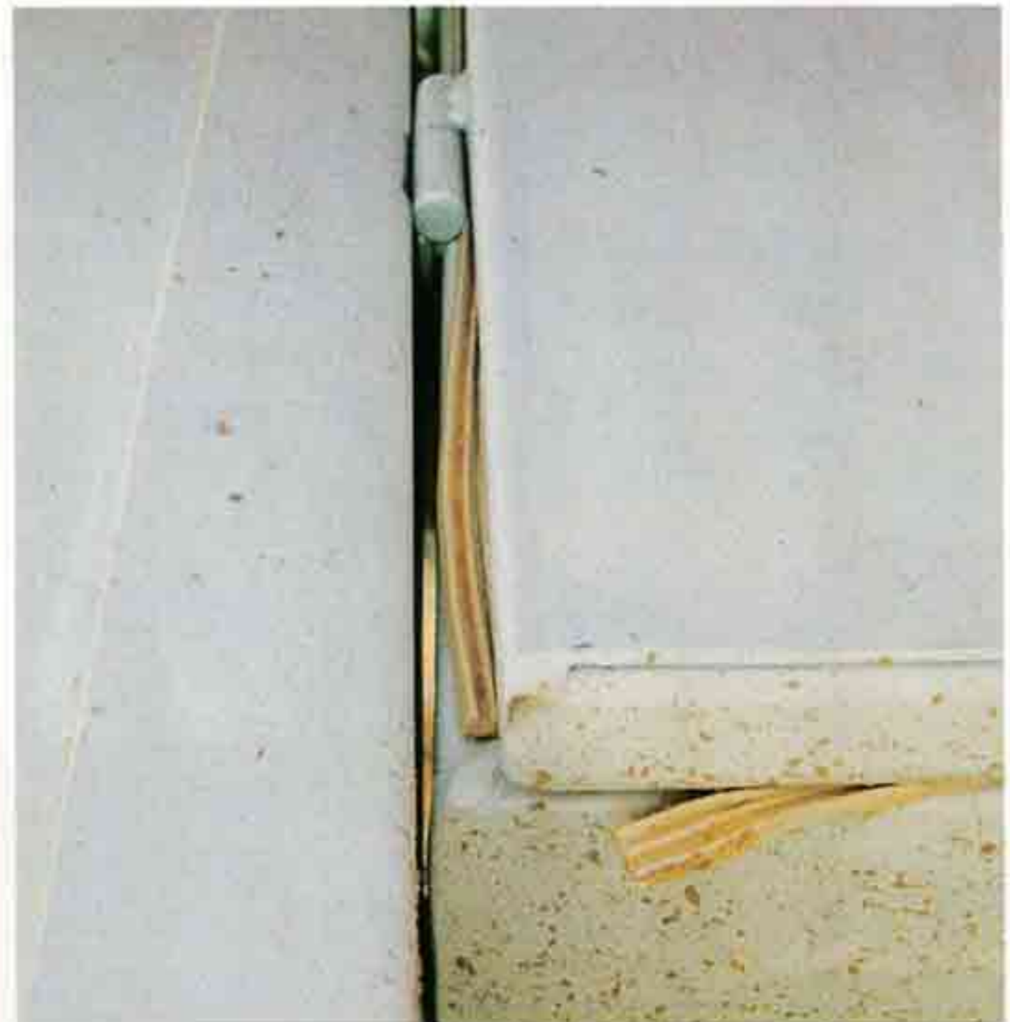
Above: How's this for a bit of dodgy sealing? Dust city, here we come!
