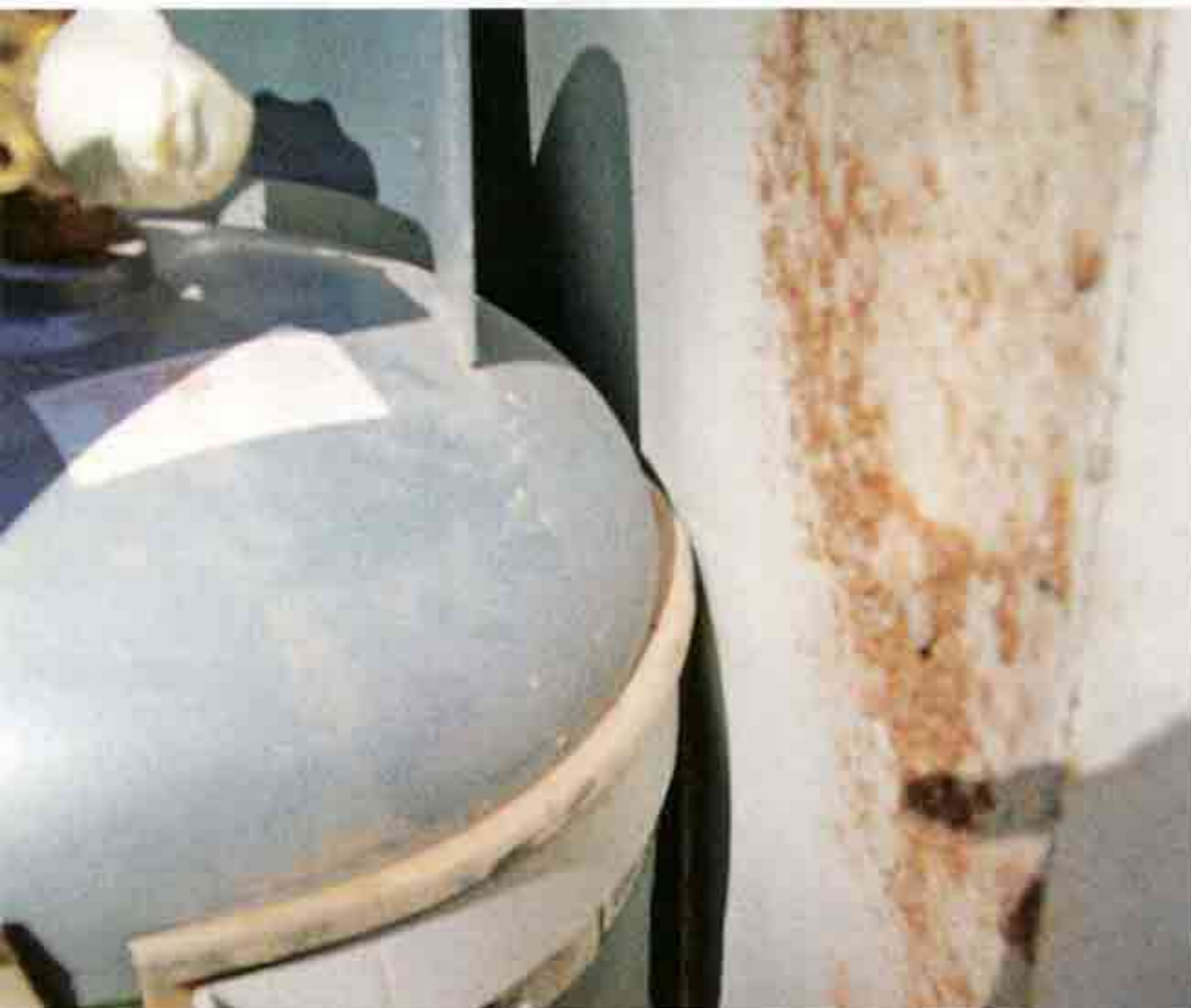
Above: Jenny [redacted] says that she and her husband had to use the gas bottle holder and jerry can holders to hold the trailer together to limp home.
